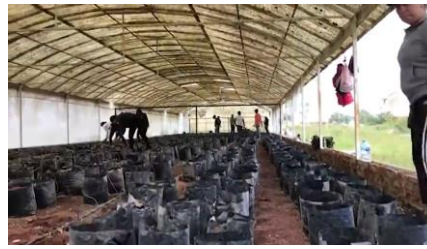
Figure 3. Rehabilitation of the greenhouses in Week i 2018 at San Luis de la Paz, Gto. (Own source)
